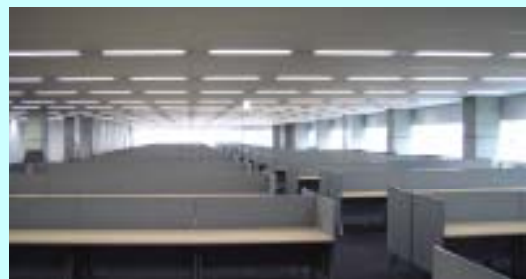
Automatic Lighting Control System
