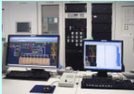
Energy Monitoring System
